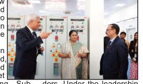
Delhi Chief Minister Rekha Gupta inaugurating a new state-of-the-art Electric Receiving Sub-Station (RSS) at Park Street.
